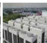
Outdoor units on the roof
